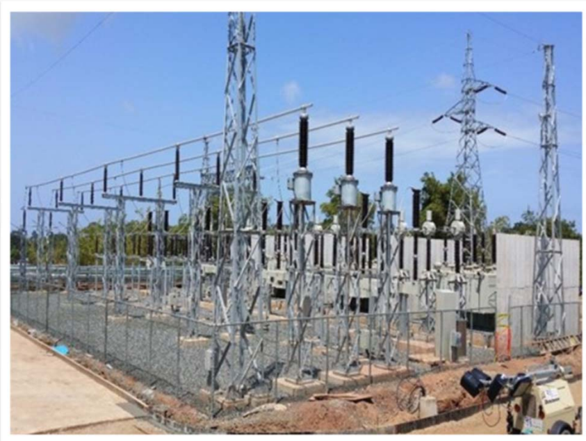
115kV Substation for JINRO Power 57.8MW PPS
