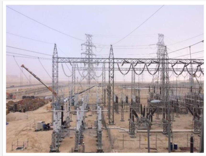
Uthmaniyah Gas Plant (UGP)
