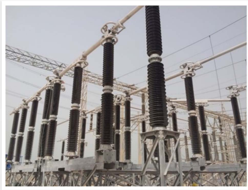
Ju'aymah Gas Plant (JGP)
